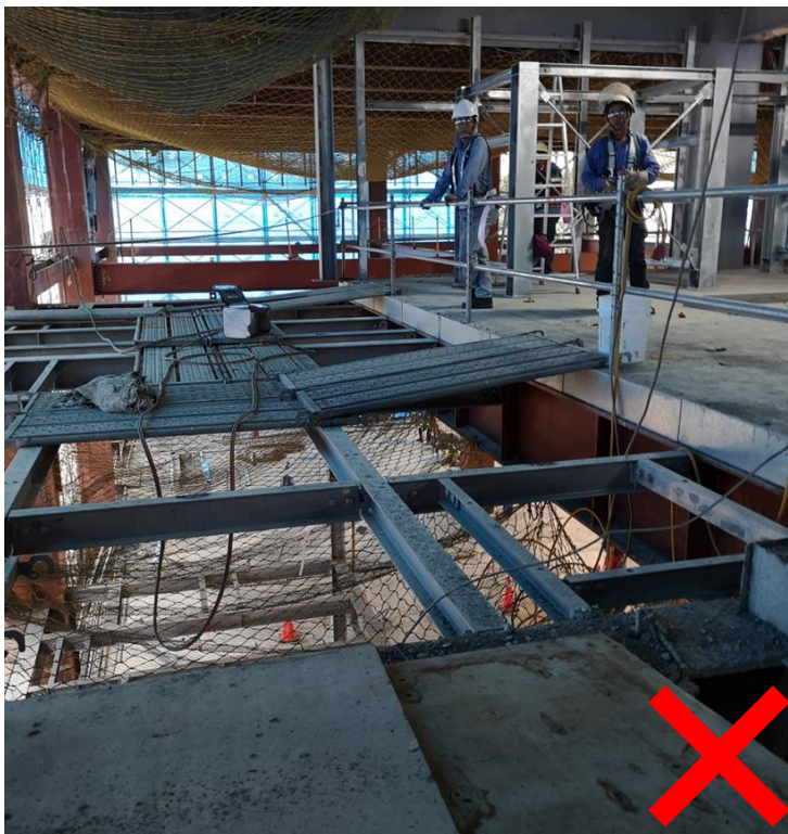
Unsafe: Platforms access to work areas do not have guardrail and lifeline
