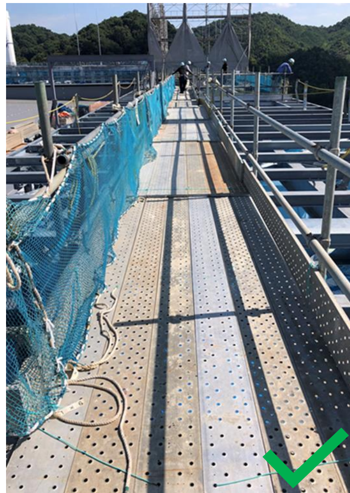
Best Practice: Proper walking platform with guardrails leading to the work areas
