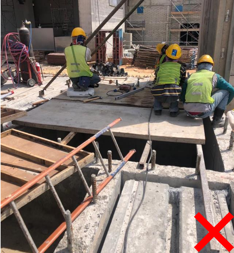
Unsafe: Hole opening covered with unsecured platform and exposed to falling hazard
