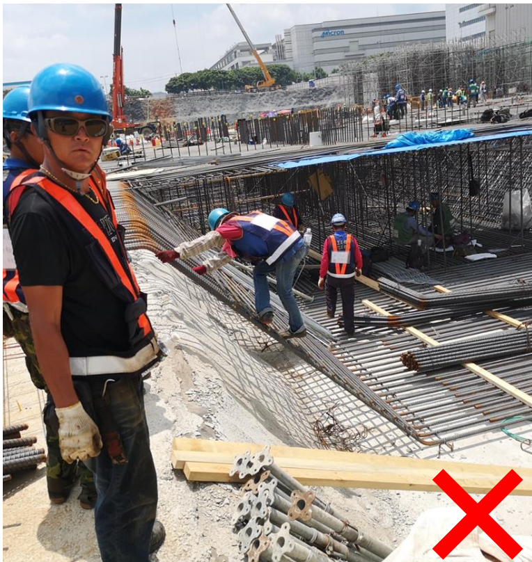
Unsafe: Workers using re-bars and timbers as alternative methods for access to work areas
