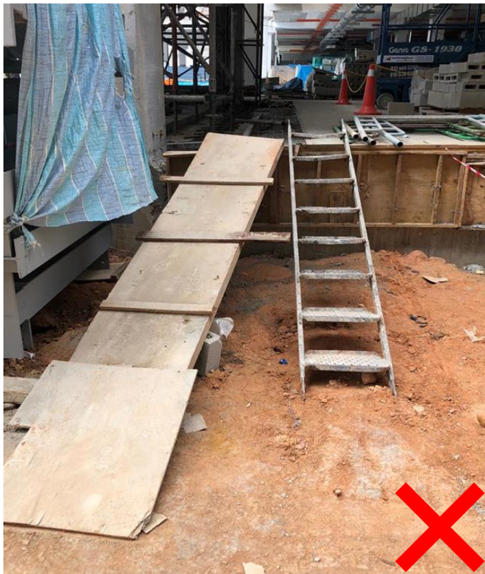
Unsafe: Makeshift timber platform and scaffold ladder used as access and egress
