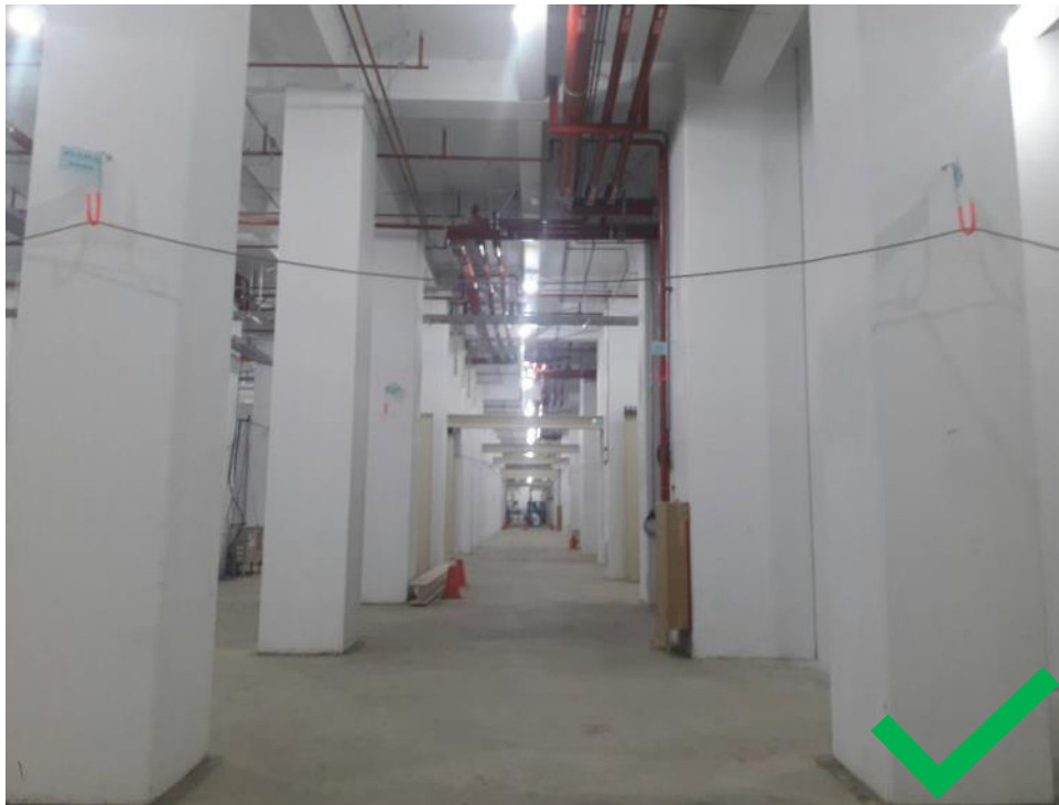
Best Practice: Electrical cables hang above 2 meters at areas used for access and egress
