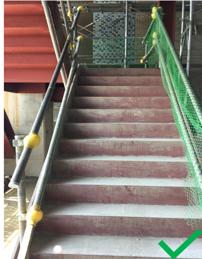
Best Practice: Stairway installed with proper guardrails and clear of tripping hazard
